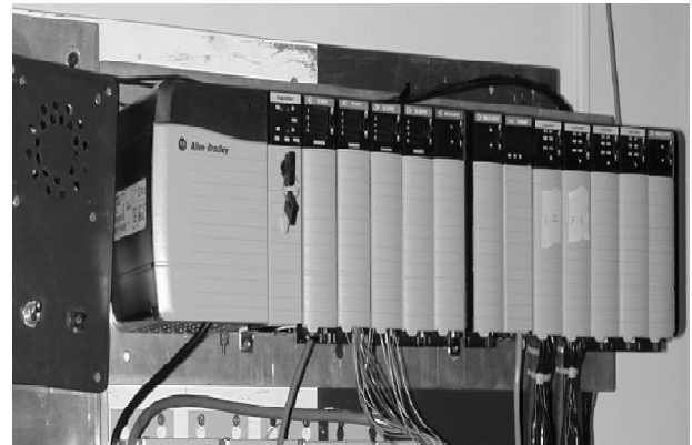
Figure.8 Allen Bradley micrologix 1200 PLC
