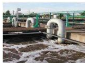
Figure.9. View of Sewage treatment plant at Hussain sagar lake
