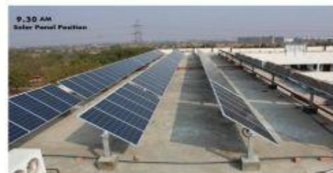
Figure 5. Single axis Tracking-Position of panels at 9:30 A.M
