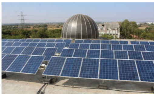
Figure 2. 20kWp Solar PV Plant on EEE Block of CVR College of Engineering
