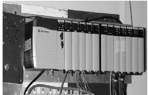
Figure.8 Allen Bradley micrologix 1200 PLC
