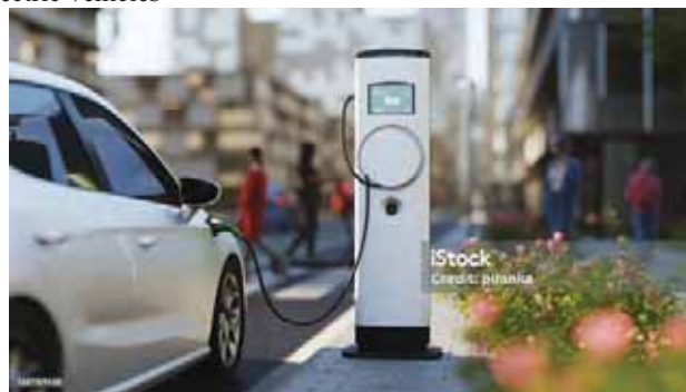
Fig 3. DC Fast Charging Station
