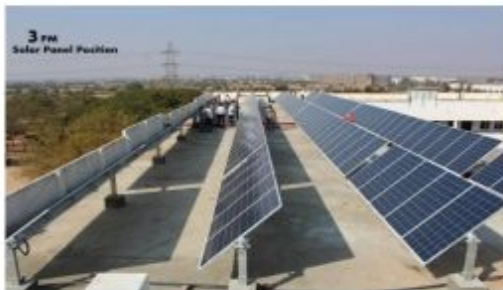
Figure 6. Single axis Tracking-Position of panels at 3:00 P.M
